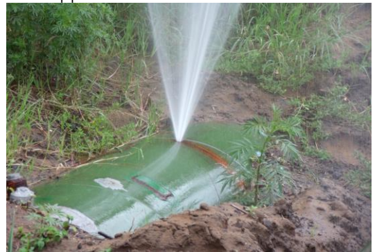
Pipe failure due to corrosion
