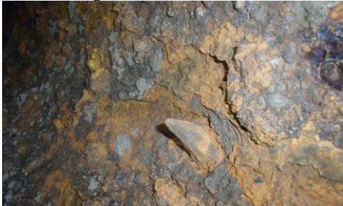
Internal corrosion of pipe
